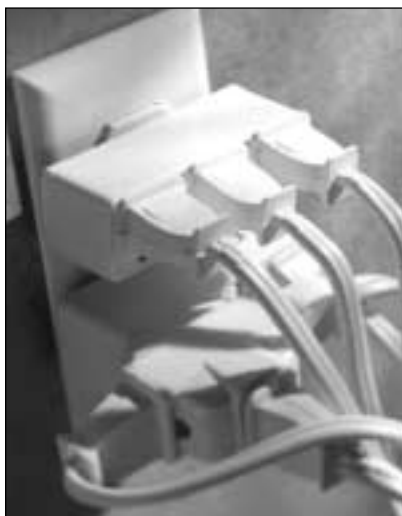
An overloaded outlet can overheat and potentially create an electrical fire.
